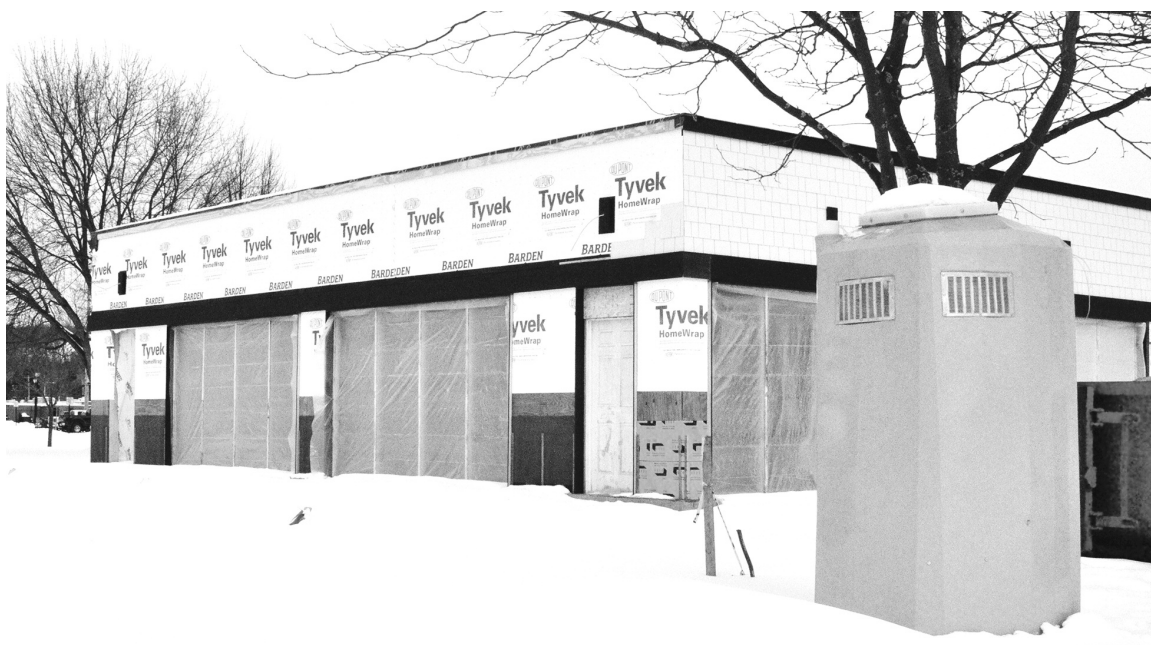
City officials have voted to move forward with funding phase two of the Veterans Memorial Park pavilion project, which will bring new bathrooms to the facility that's been under construction for the past several months. PHOTO BY MICHELLE MEDJESKY;
